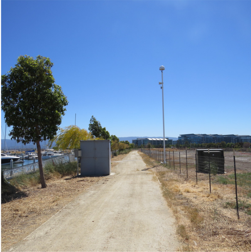
1 Figure 22 - PG&E Box Near Path 413
